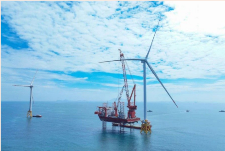
Illustration (Photo: Jiangsu Hengtong Optic-Electric)
