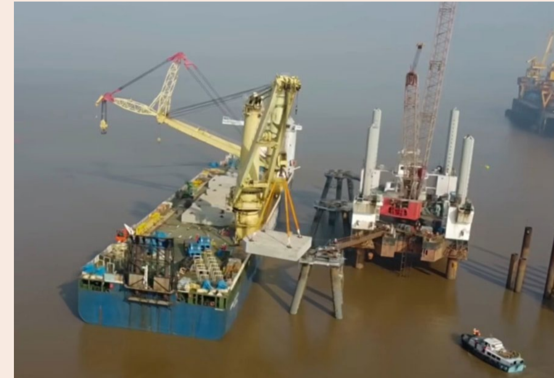
Heavy-lift installation operations for the GCPL berth project in India. The image was captured from a LinkedIn video posted by JSI Alliance.
